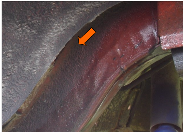
Visible sound deadener overspray on the frame rail though exterior paint has worn off.
